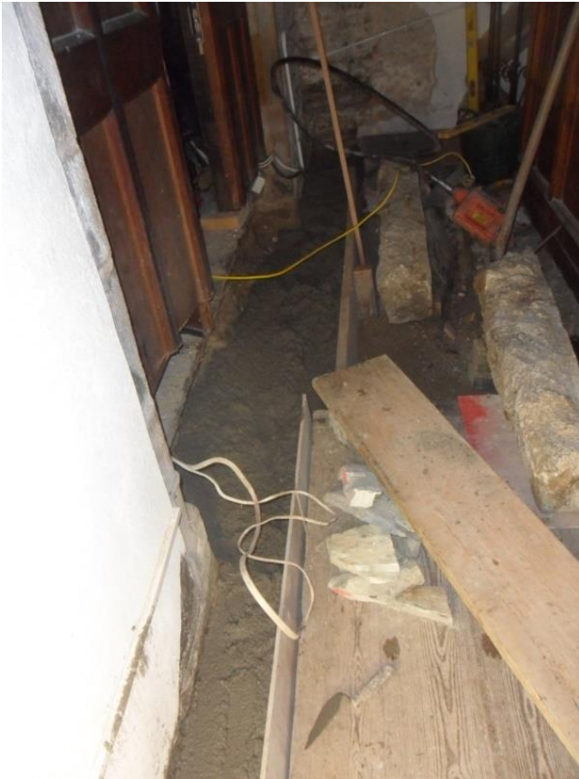
THE GRANITE STEPS TAKEN OUT AND A NEW CONCRETE BED FORMED THIS REQUIRED THE DISMANTLING OF THE BASE OF THE SCREEN, THIS HAS NOW BEEN REPAIRED
