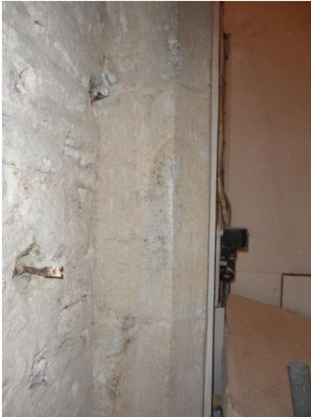
CORODING IRONWORK BEDDED INTO THE TOWER NORTH WALL, THERE IS ALSO SOME IN THE SOUTH WALL
