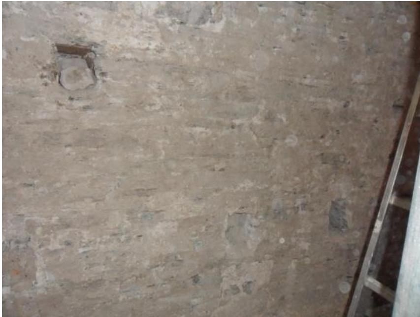
AFTER REMOVAL OF THE RENDER ON THE TOWER WALLS PATCHES OF LIME PLASTER ARE STILL EVIDENT ON THE WALLS SHOWING THAT THIS WAS THE ORIGINAL FINISH BEFORE THE HEAVY CEMENT MORTAR WAS APPLIED
