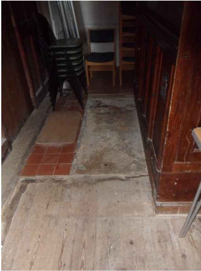
BEFORE START OF WORK TO CREATE THE NEW GULLEY TO HOLD THE ELECTRICAL WIRING
