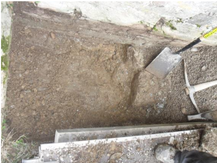
EXTERNAL TRENCH ON THE SOUTH SIDE OF THE TOWER, THIS HAS BEEN EXCAVATED DOWN TO THE BED ROCK ON WHICH THE TOWER HAS BEEN BUILT AND IS NOW BEING REFILLED WITH STONES TO DRAIN MOISTURE AWAY FROM THE BASE OF THE WALL
