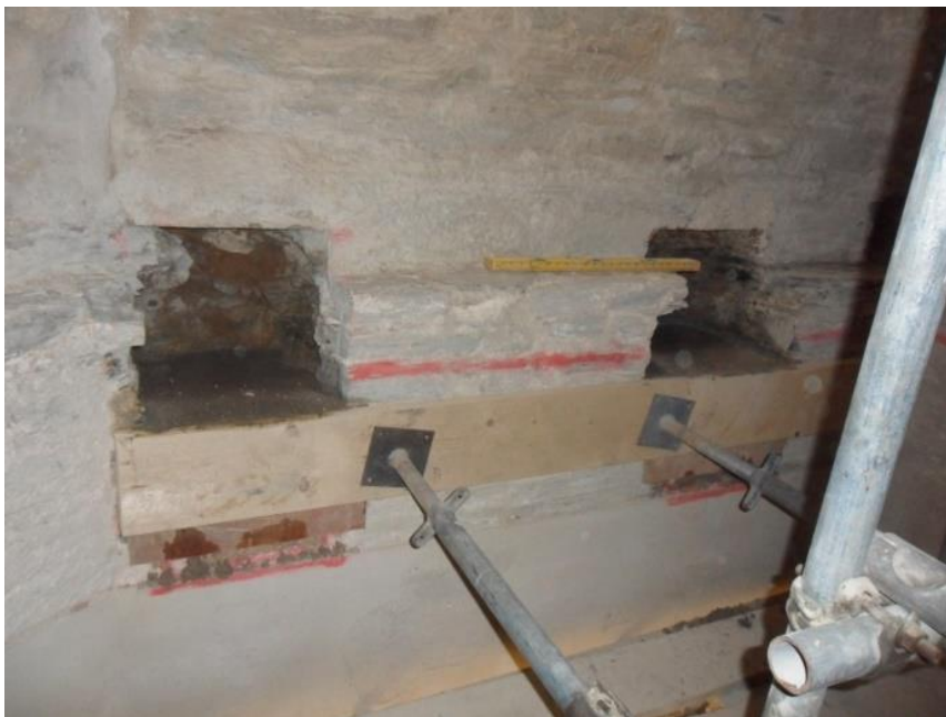
CONCRETE PADSTONES FOR THE NEW BELL FRAME CAST IN THE NEW POCKETS IN THE NORTH WALL
