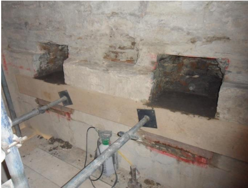
CONCRETE PADSTONES FOR THE NEW BELL FRAME CAST IN THE NEW POCKETS IN THE SOUTH WALL
