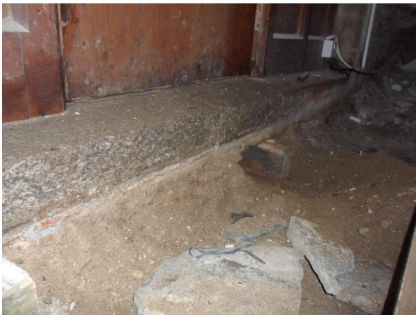
DURING THE EXCAVATION WORK IT BECAME CLEAR THAT A PROPER BED FOR THE STEPS HAD NEVER BEEN CREATED CONSEQUENTLY THEY ROLLED FORWARDS
