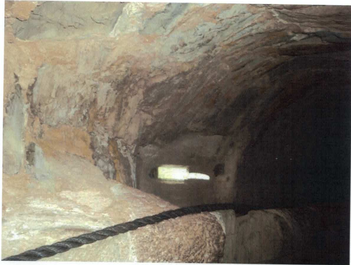
STAIR WINDOW AND CRACKED LINTEL BEFORE REPAIR
