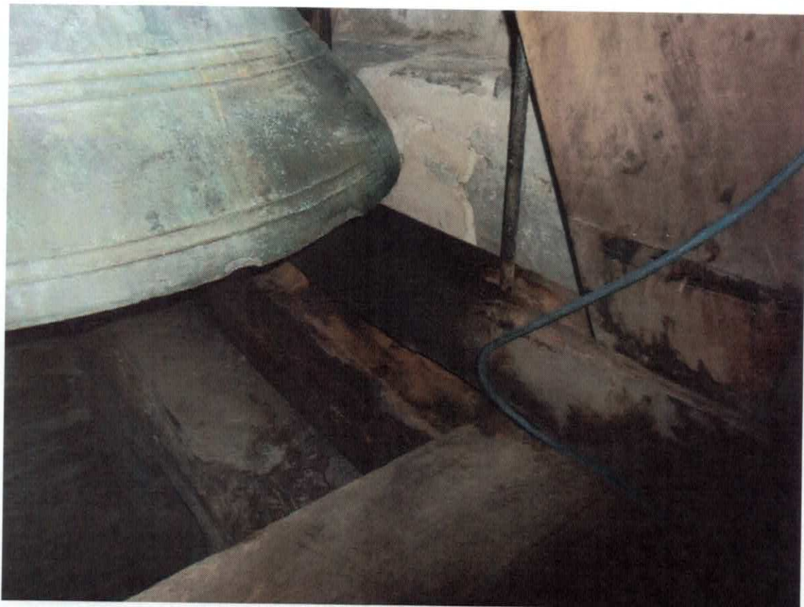
ROTTED SOUTH BEAM TO BELL CHAMBER FLOOR AND BOTTOM RAIL OF BELL FRAME.
