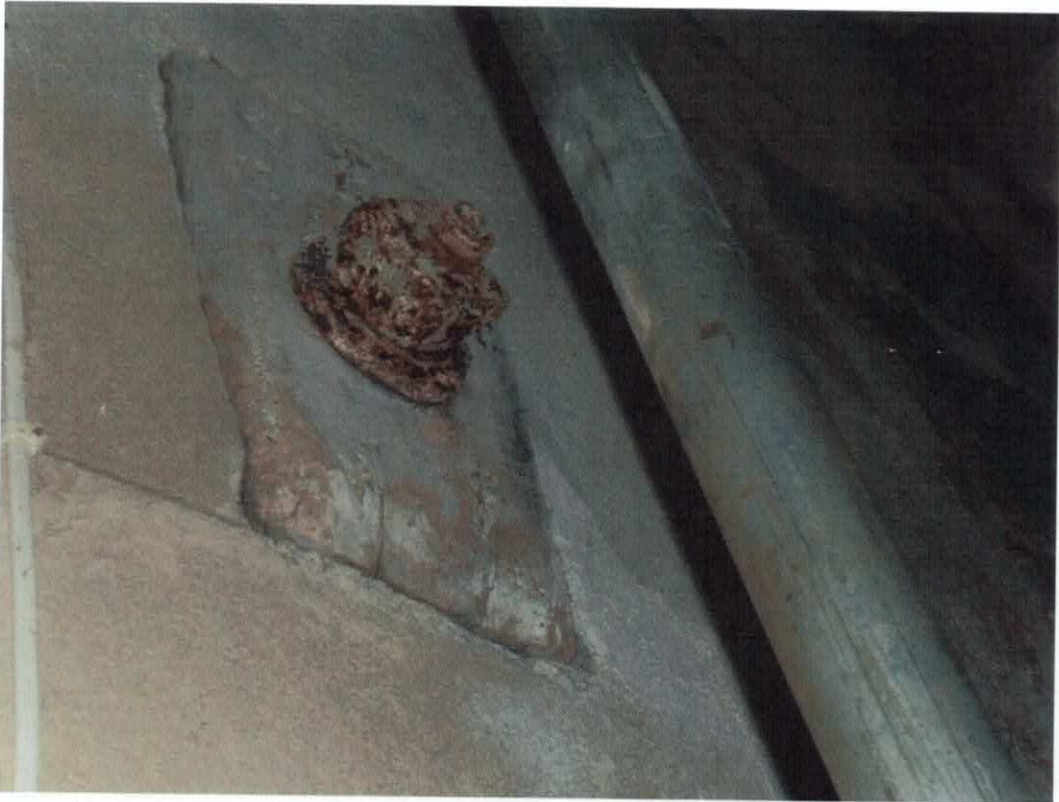
OAK PAD TO BOLT TO NAVE ROOF, EXISTING PAD IS ROTTEN AND HAS WOODWORM.
