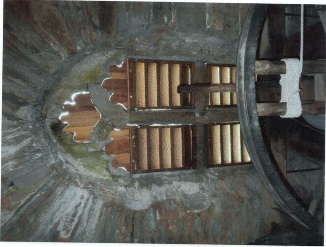
SOUTH BELL CHAMBER OPENING BEFORE REPAIR
