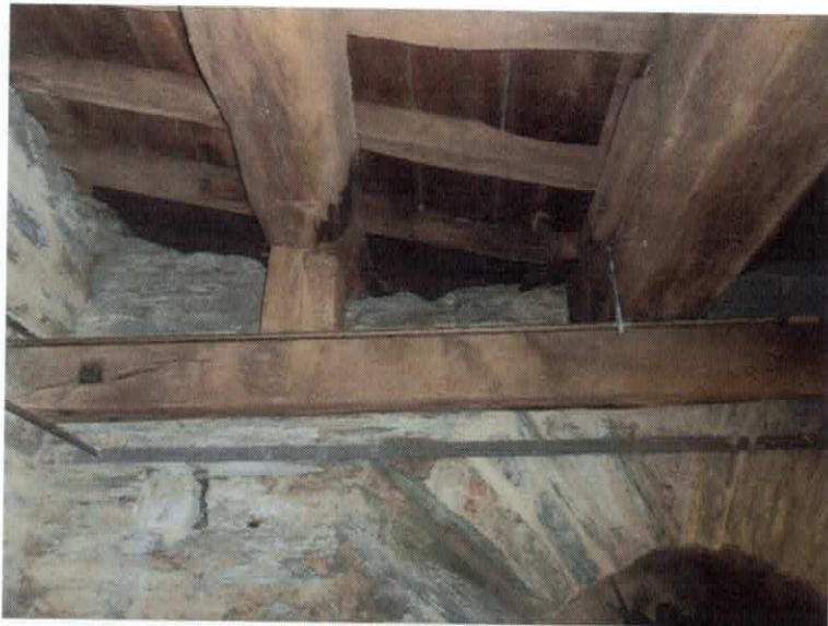
NEW OAK BLOCK, MADE TO FULLY SUPPORT THE EASTERN ROOF BEAM FROM THE EAST END OF THE SOUTHERN TIE BEAM.
