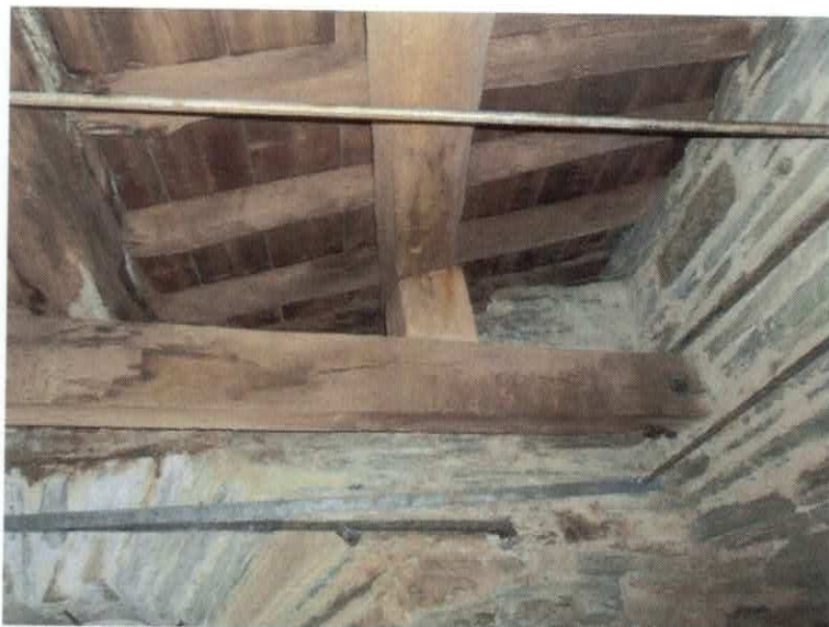
NEW OAK BLOCK MADE TO SUPPORT THE NORTHERN END OF THE EASTERN ROOF BEAM FROM THE EAST END OF THE NORTHERN TIE BEAM. THERE WAS NO BLOCK HERE BEFORE WORKS STARTED. THE YEAR 2016 HAS BEEN CARVED INTO THE SOUTHERN SIDE OF THIS BLOCK.
