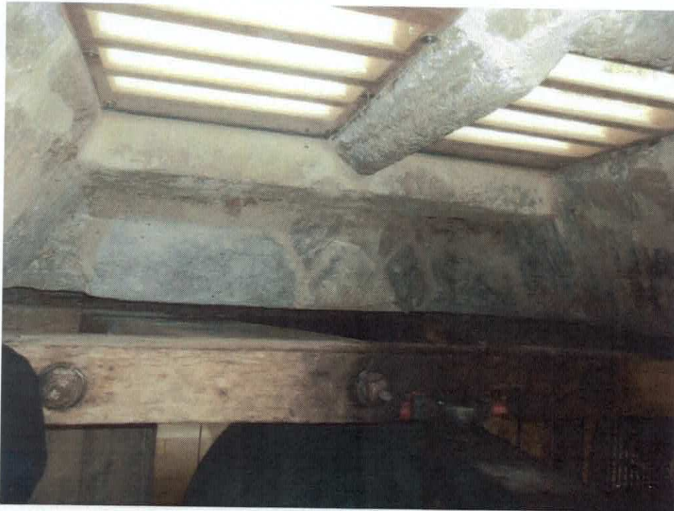
SOUTH BELL CHAMBER WINDOW LEDGE AFTER RUBBLE REMOVAL AND CLEANING DURING FIRST PHASE – 6 WHEELBARROW LOADS OF RUBBLE, DUST AND BIRDS NESTS WERE REMOVED FROM THE BELL CHAMBER, LARGELY FROM AROUND THE EDGES OF THE BELL FRAME BUT ALSO FROM THE TOPS OF THE WALLS
