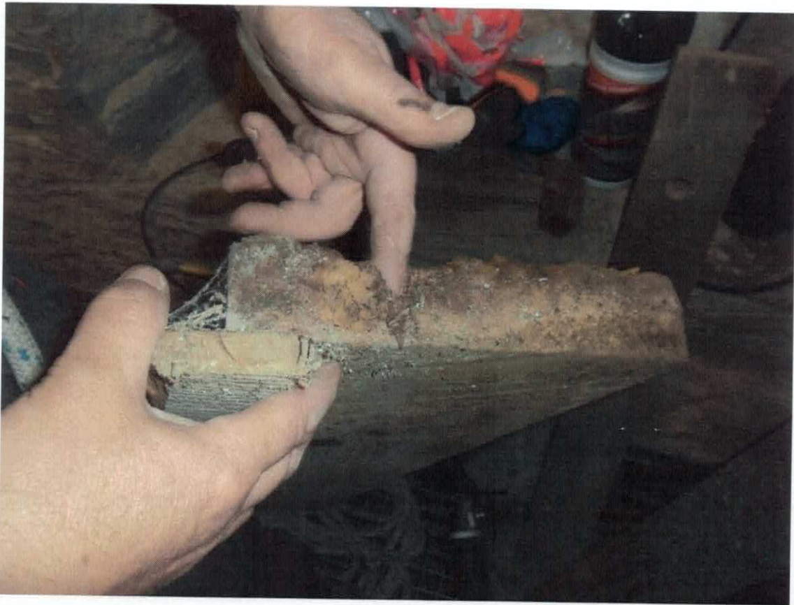
ROTTEN BOARDS WHICH FORMED THE HATCH UNDER THE TENOR BELL, NORTH SIDE WERE ROTTEN AND SOUTH SIDE ONLY JUST RESTING ON A ROUNDED BEM EDGE.
