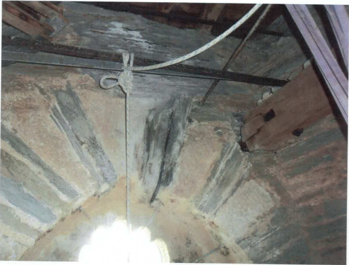
BELL CHAMBER WEST WALL BEFORE REPAIR
