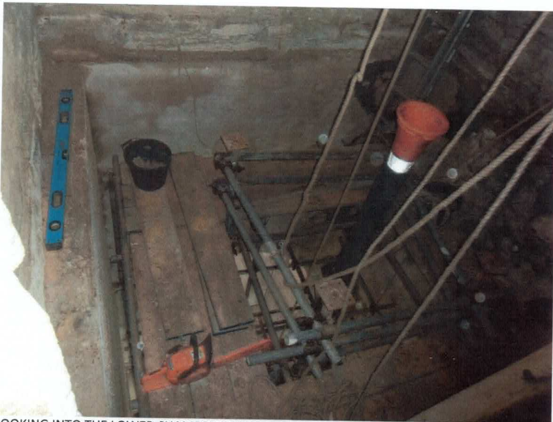
LOOKING INTO THE LOWER CHAMBER SPACE FROM THE STAIR DOORWAY AFTER REMOVAL OF THE ROTTEN FLOOR
