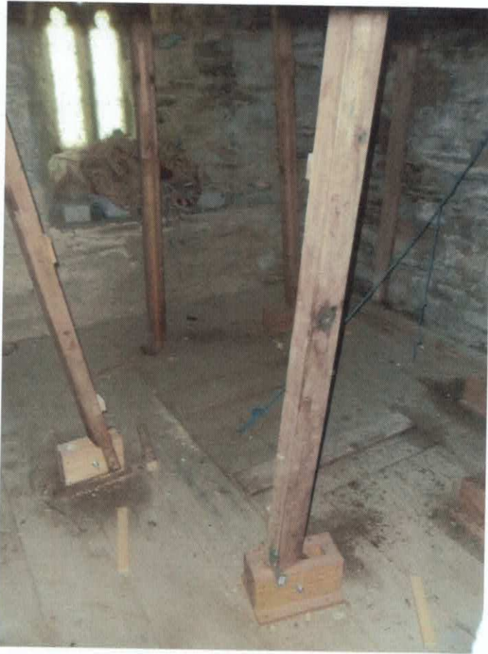
LOOKING INTO THE LOWER CHAMBER FROM THE STAIR DOORWAY BEFORE REMOVAL OF THE ROTTEN FLOOR
