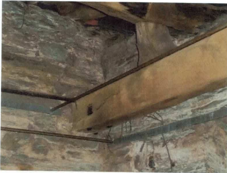
OLD ROTTEN BLOCK (SECTION OF TREE TRUNK) TO EAST END OF SOUTHERN TIE BEAM.
