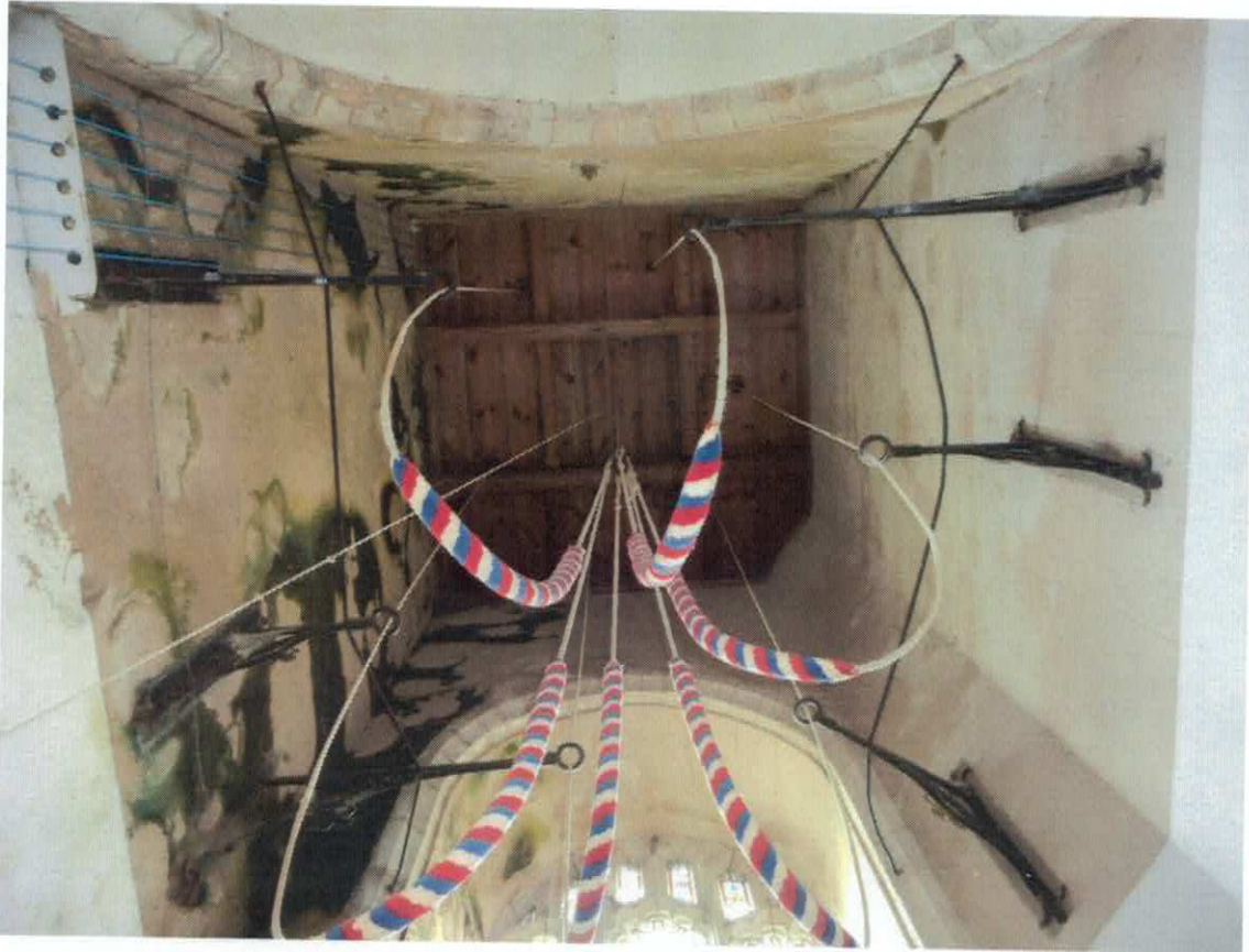
LOOKING UP INSIDE THE TOWER TO LOWER CHAMBER FLOOR BEFORE THE REMOVAL OF THE ROTTEN FLOOR.
